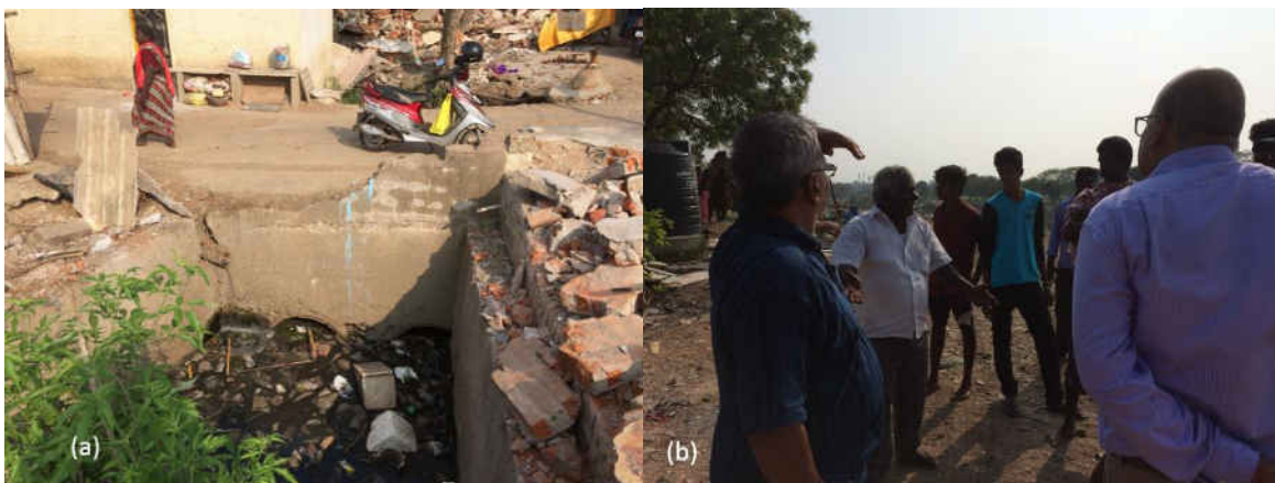
Figure 27: (a) Poor condition of storm water drainage near Adyar River, Ferry Road, (b) Feedback being received from the local residents.
